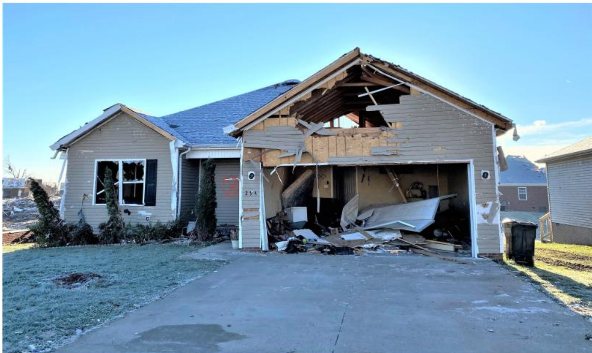
Figure 7. Loss of roof sections and gable end framing initiated from garage door failure Bowling Green, Kentucky (December 2021)
