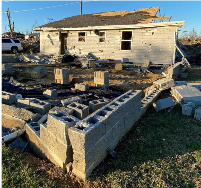
Figure 1. Failure of load path, building envelope components (roof shingles, soffits, and siding) and windows observed in Dawson Springs, Kentucky (December 2021)
